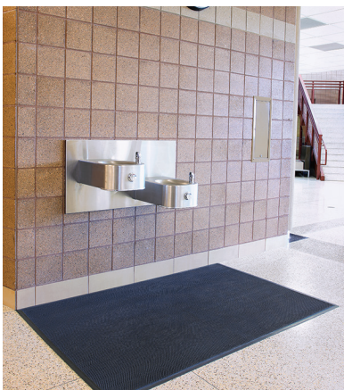
DRINKING FOUNTAINS & WET AREAS
